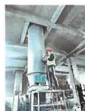
◎3DA003 2#包装机排放口 3#
